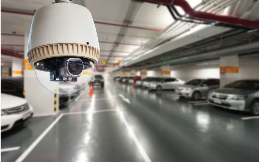
Figure 8: Installing surveillance cameras in public car parks can discourage vandalism.
